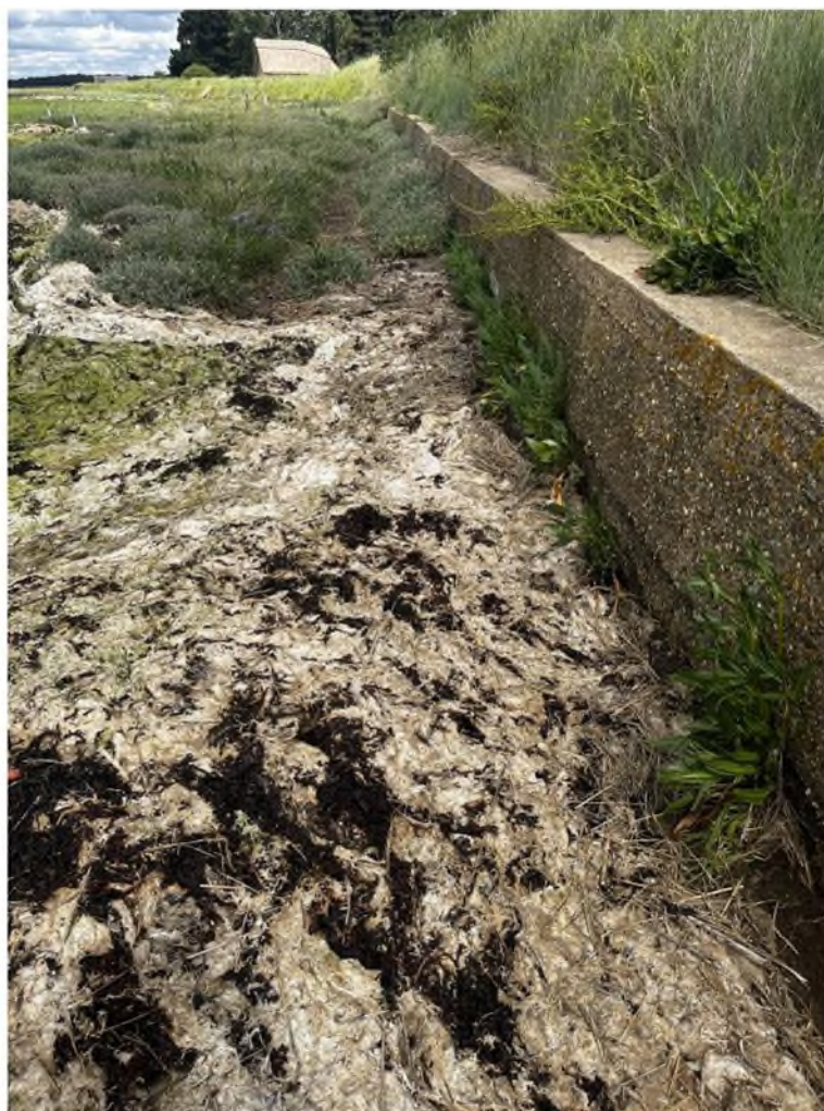
High tide debris to to concrete wall
