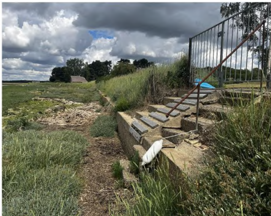
High tide debris up to concrete wall
