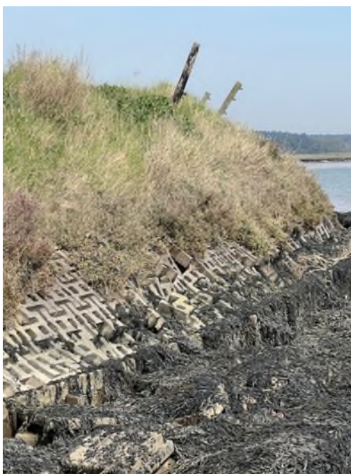
Pic 9 - High water continues to damage the armour on the corner opposite Dove Point
