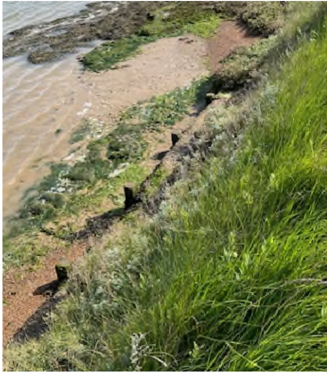
Photo 9 – Overtopping occurring to previously repaired river wall between Dove Point and the Butley river
