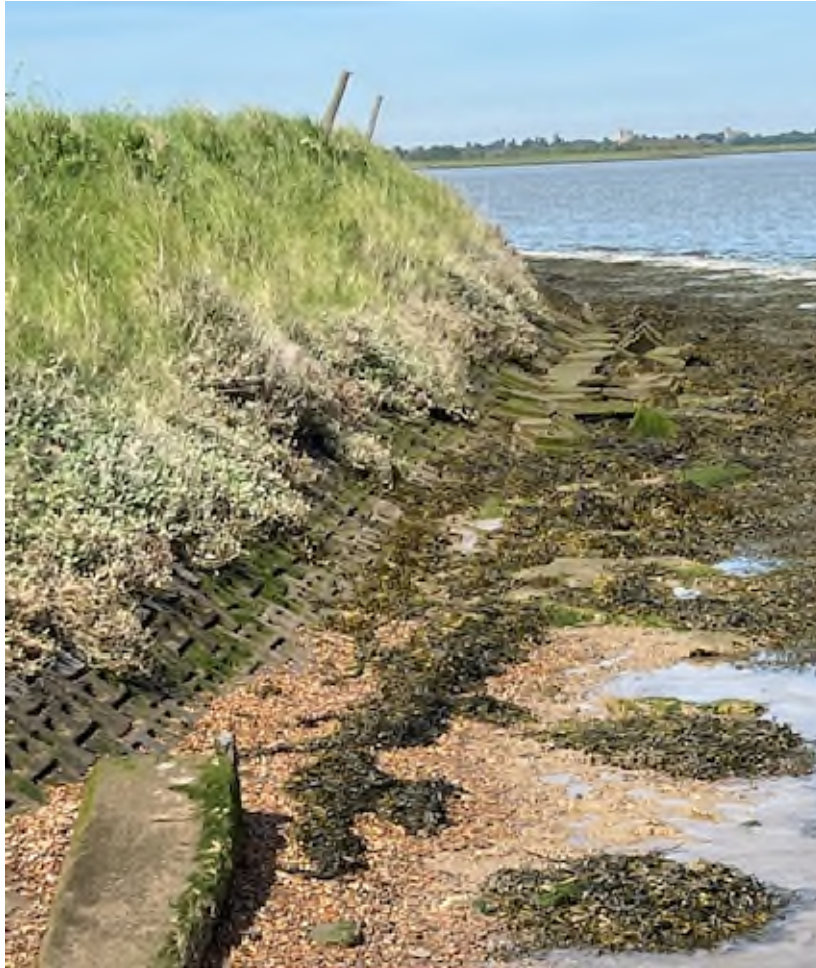
Photo 7 – Grid reference 52°03.920'N, 1°29.758'E – Dove Point - showing extensive signs of wear
