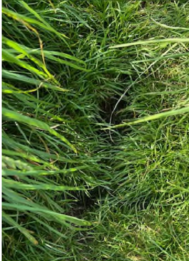
Photo 13 - grid reference 52°04.251'N, 1°29.745'E. – quite a few ‘Sink holes’ appearing between Butley entrance and Boyton dock. A lot hidden by vegetation.
