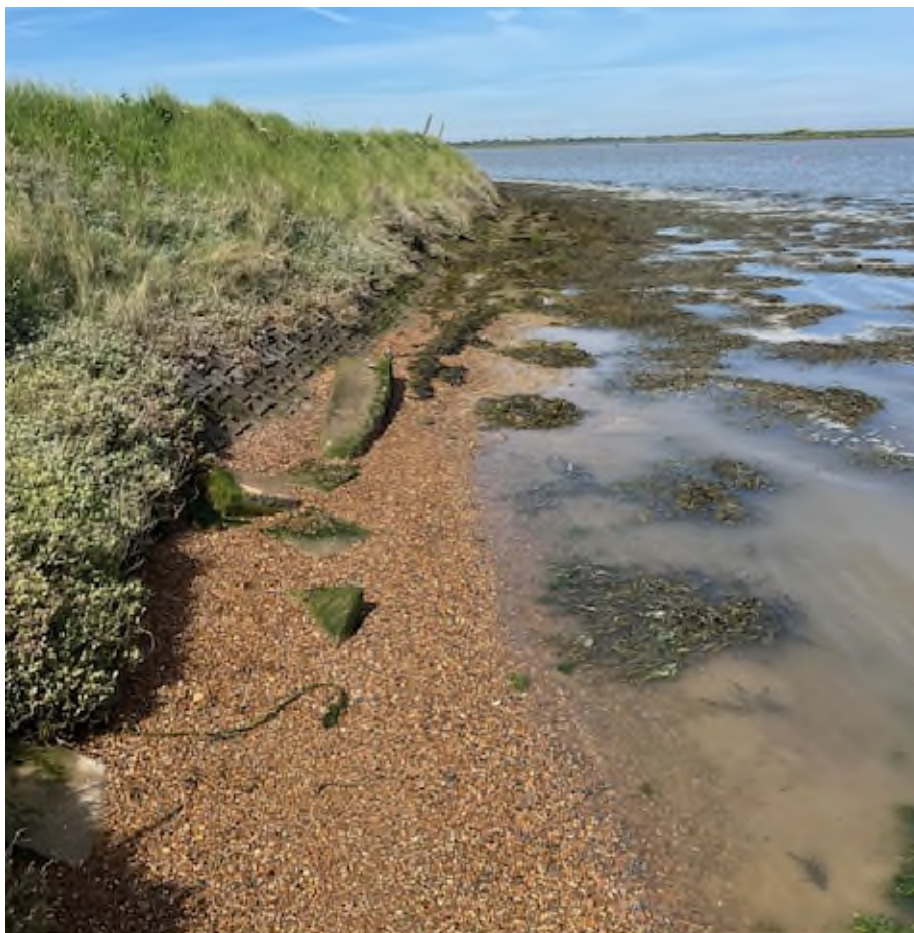
Photo 6 – Grid reference 52°03.920'N, 1°29.758'E – Dove Point - showing extensive signs of wear
