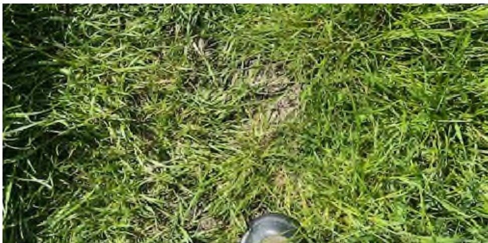
Photo 12 – Grid reference 52°04.251'N, 1°29.745'E. - Cracking appearing between Butley entrance and Boyton dock
