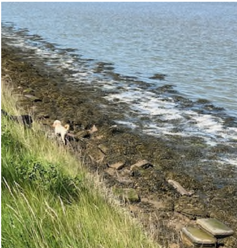
Photo 8 – Grid reference 52°03.920'N, 1°29.758'E – Dove Point - showing extensive signs of wear
