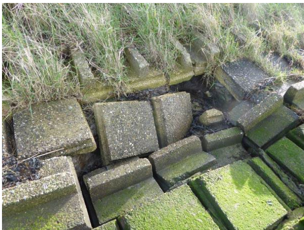
Image: Damaged block revetments to be repaired
