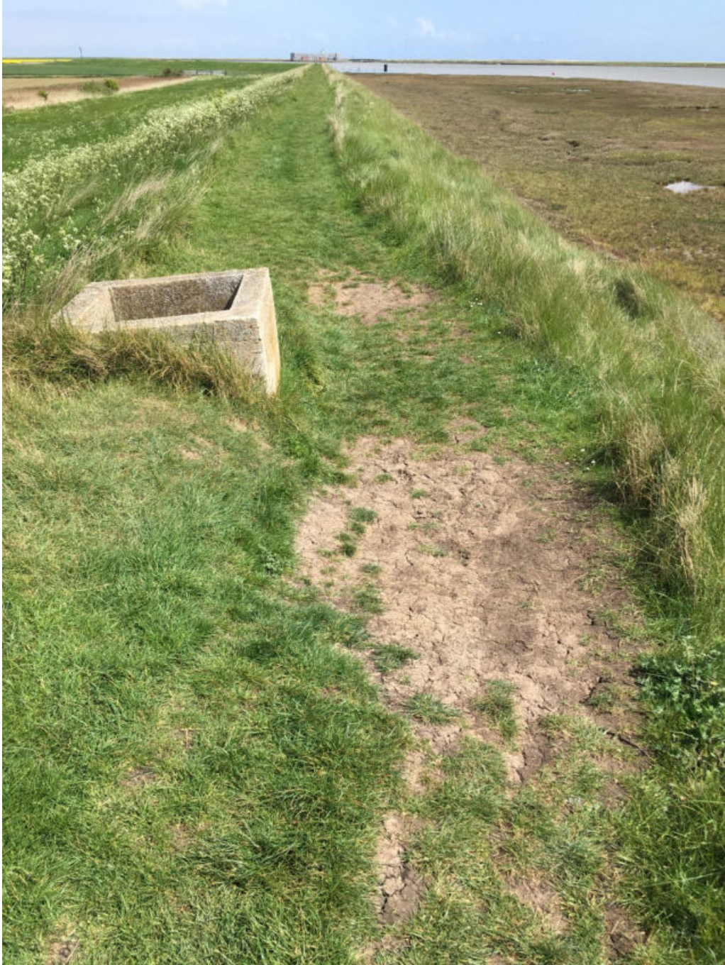
Dip in wall getting bigger [437 500]
