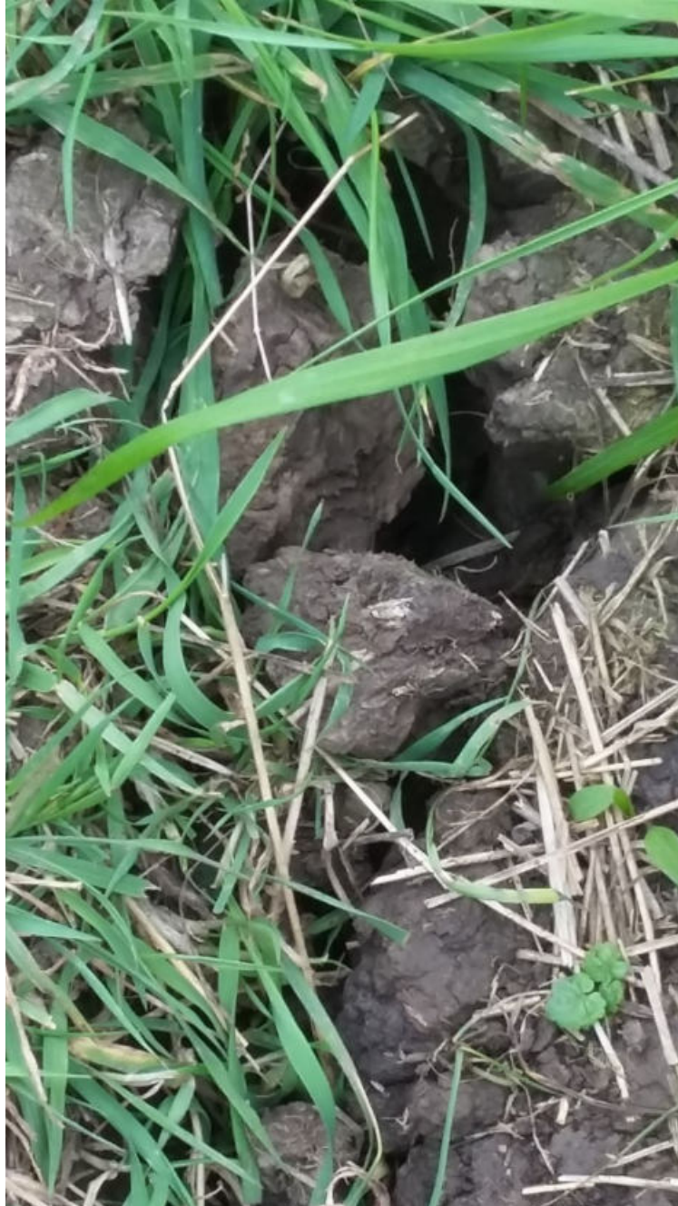
Photo 1 – Cracking in side of wall by sewage outlet
