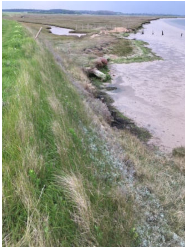
Chainage 4000 to Boyton Dock: Top of wall uneven with some cracking, and increased undergrowth due to lack of grazing (Photo 6)
