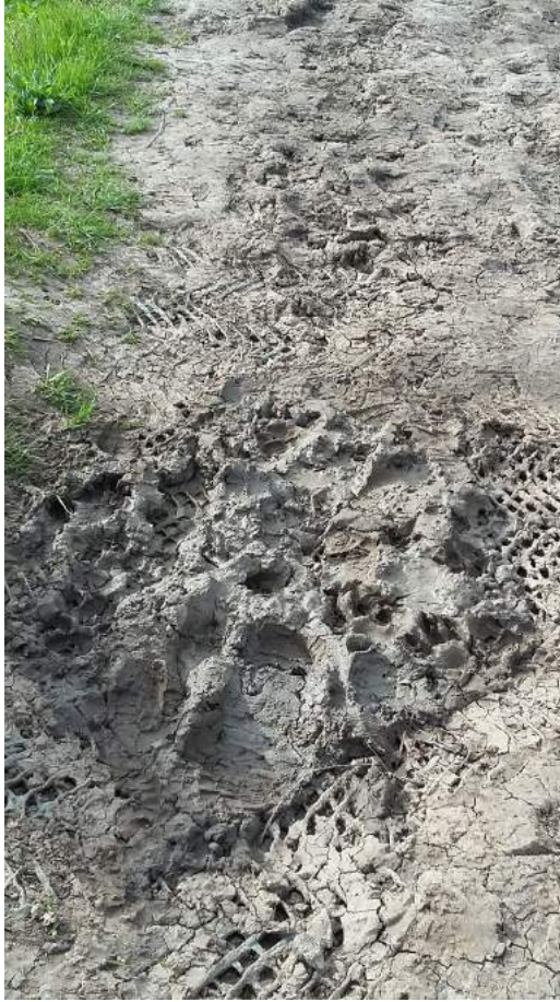
Photo 2 Surface turning to mud and exposing netting
