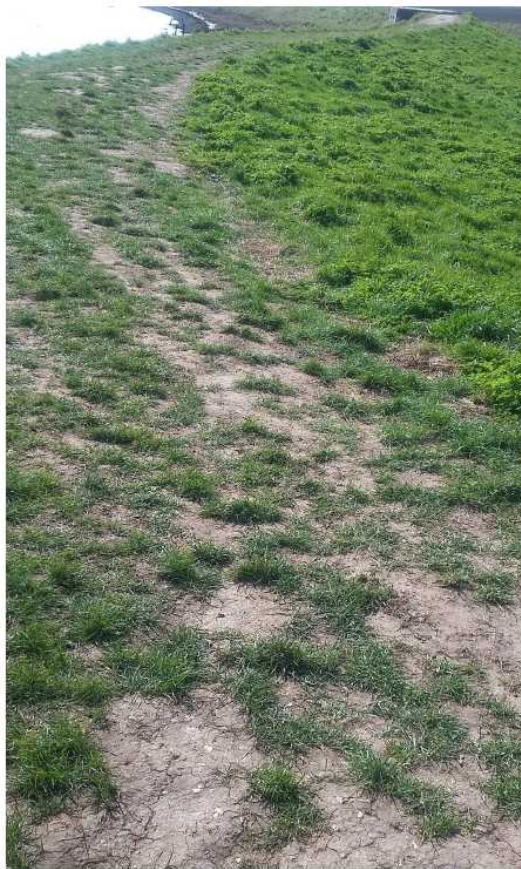
The top of the wall now has a significant slope away from the river as the wall bends toward the pillbox.
