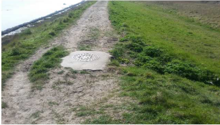
The area round the drain cover is more worn (this is of course where there was overtopping in 2013)
