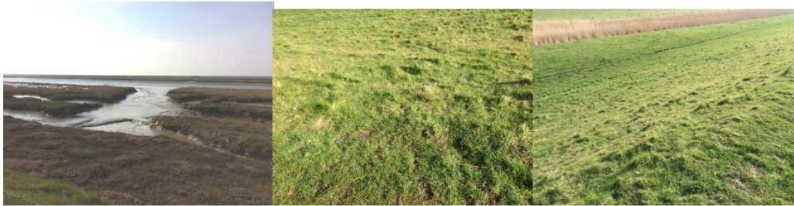
Saltings, pathway and landward wall at 394474, past Boyton Dock. Saltings unchanged, landward side and path apparently in better order than 2015, damage to path grassed over and no evidence of previous apparent slippage on landward side.
