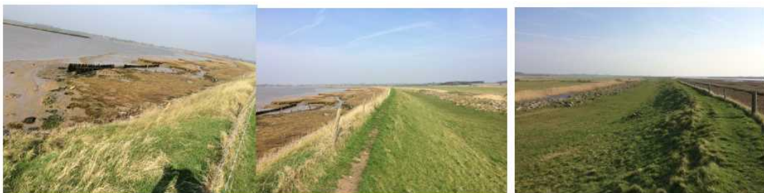
At 407471, Inset Point – saltings slightly cut away over winter (??); path still damaged and narrowed
