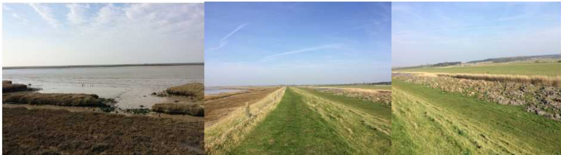
Towards Inset Point, at 405472 – saltings unchanged, path still worn and damaged but better grassed than 2015, spoil berm by ditch on landward side grassing over well.
