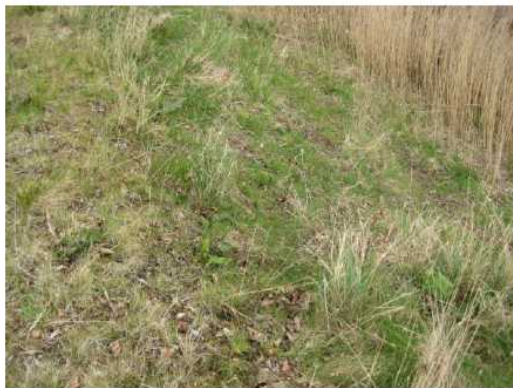
North of No1 Sluice: settlement
