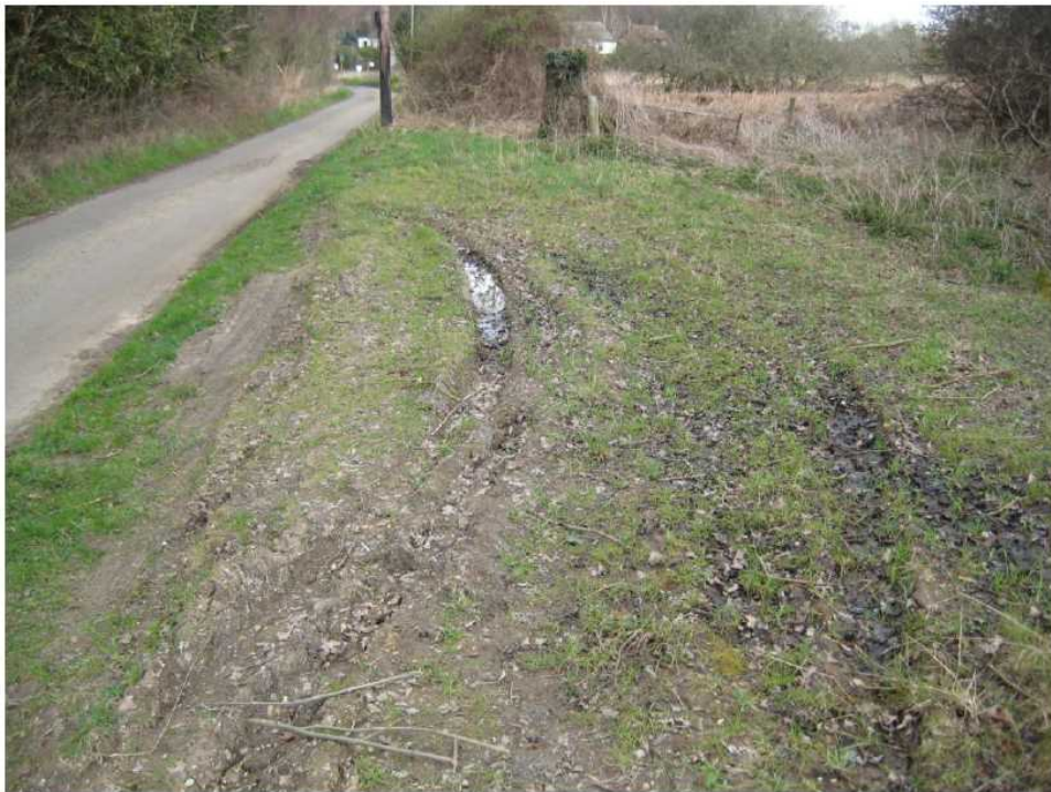
Chillesford end of wall: tyre tracks at the start of the defence.
