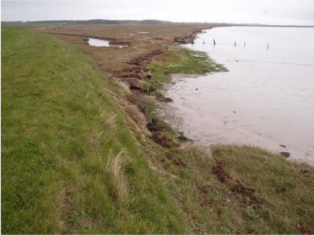
CHAINAGE 4500 2 short lengths where bottom of levee is unprotected by either salting or shingle. Long fetch of open water by south end of Havergate makes this bank vulnerable.
