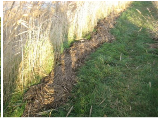
8 overtopping East wall
