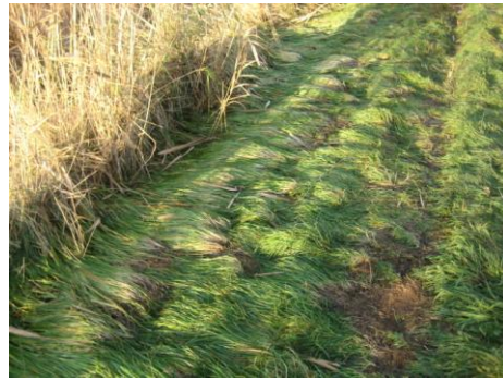
7 Overtopping East wall
