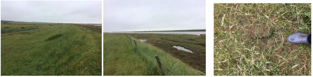
At 408 473, path towards the pumping station – landward and river-ward walls both in good condition, but some serious cracks and fissures in the path.
