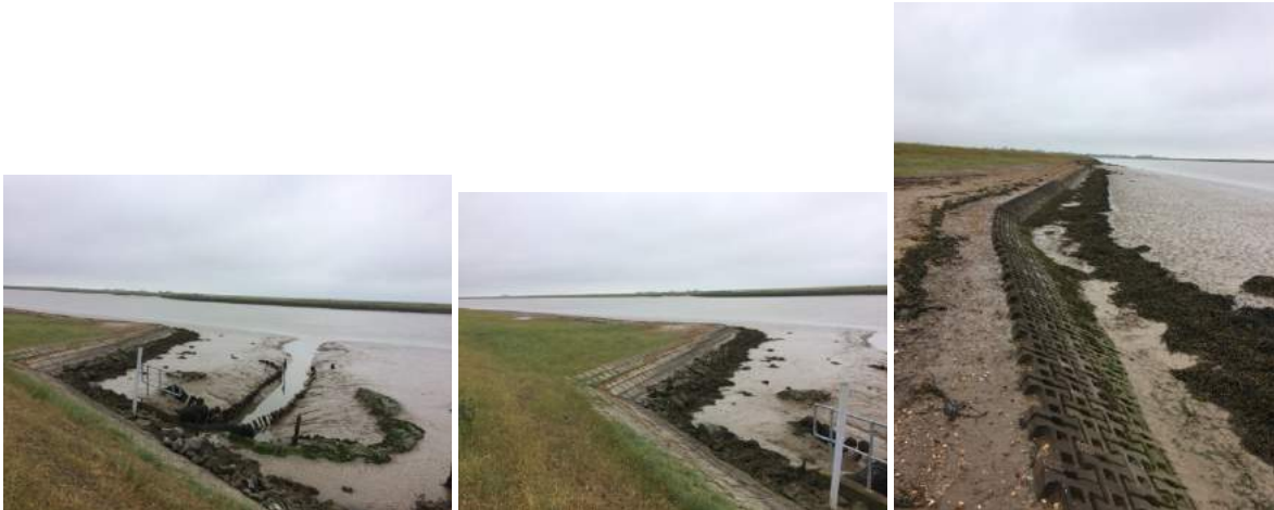
At the pumping station inlet, 411475. No significant change since 2015& 2016, river wall revetments all in good order here and further along.
