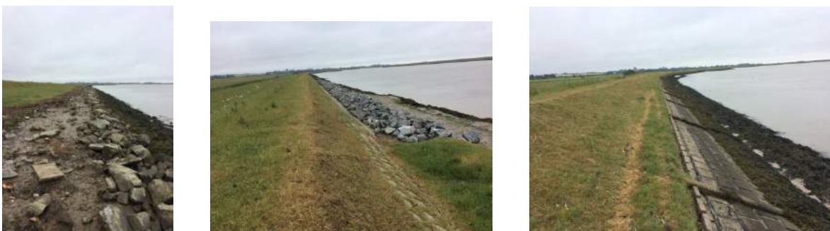
Boulder and shingle defences at 412477, revetment and (at 414 482) new lower path appearing at foot of
