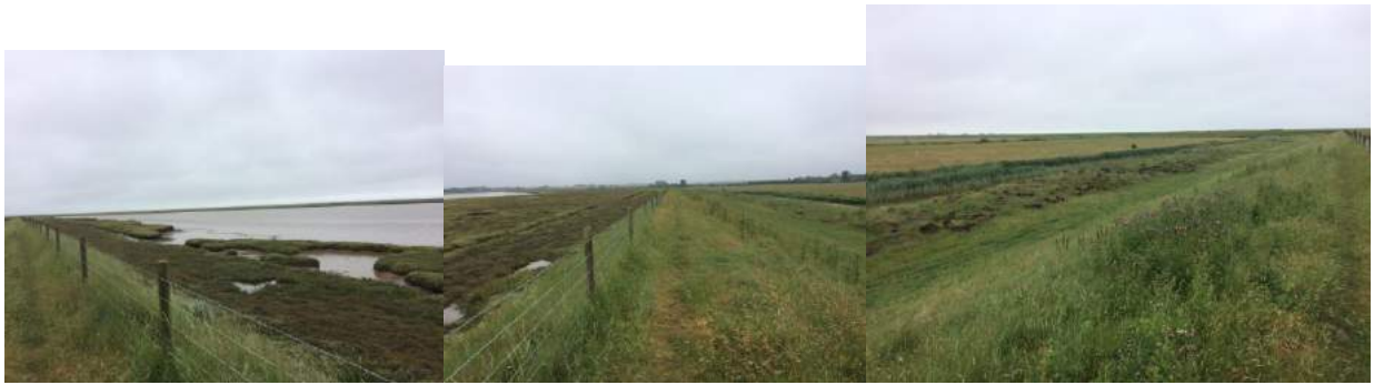
Saltings, pathway and landward wall at 406 473, past Boyton Dock. Saltings unchanged, landward side and path in good order, no evidence of previous slippage on landward side.
