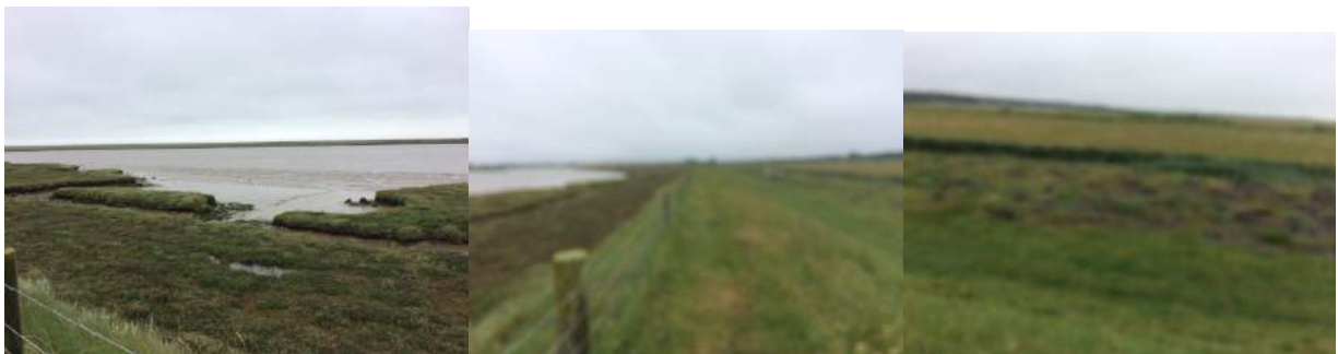
Towards Inset Point, at 405 471 – saltings unchanged, path still worn and damaged but better grassed than 2016, spoil berm by ditch on landward side now completely grassed over.
